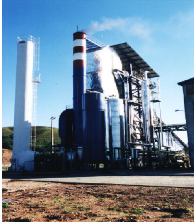
Biomass Power Generation Plant
